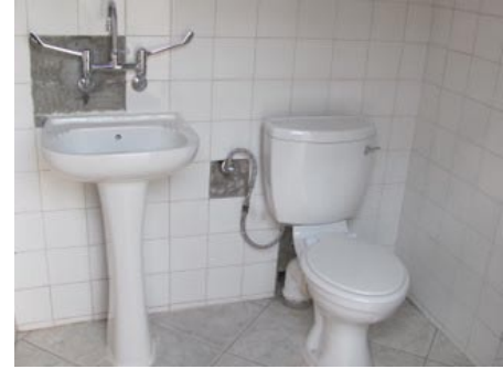
Sinks and toilets imported from South Africa being installed in the hospital
