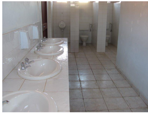
Men's ablution block
