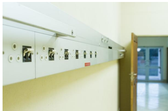
Sophisticated over bed units in the ICU with piped in oxygen, suction, power, lights – donated by Pretoria hospitals and installed throughout the complex
