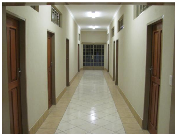
View into the clinic corridor – consultation rooms, pharmacy, laboratory, minor surgery, etc.
