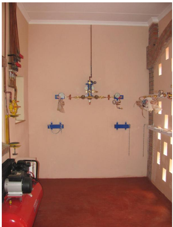
Utility area – source of piped in oxygen, suction, compressed air, and surgical gases
